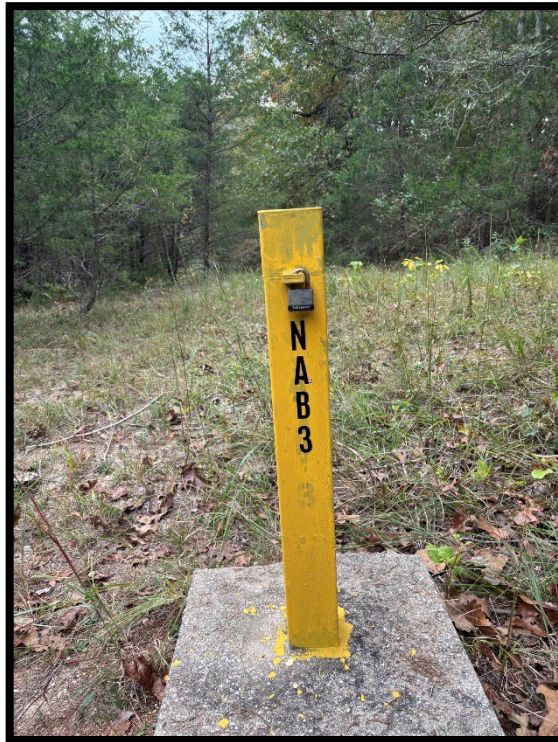
Photograph 8: View of re-labeled stickup at NAB-3.
