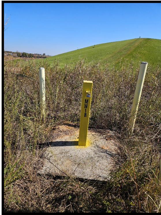
Photograph 3: View of re-painted and re-labeled stickup at MW-1R.
